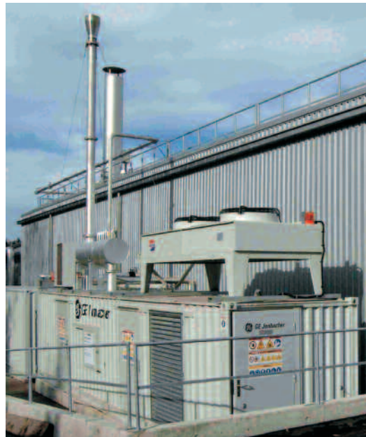
Fig 3 Typical containerised CHP unit for biogas
