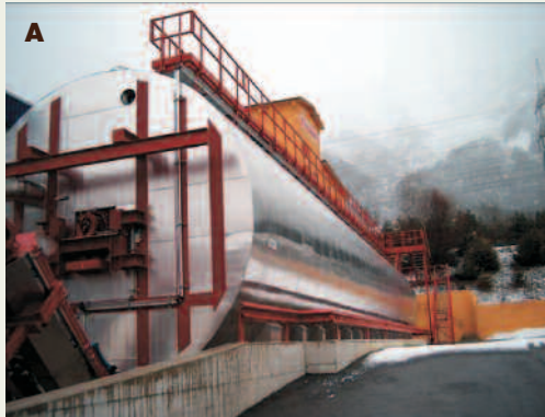
Fig 6 A selection of anaerobic digestion plants
